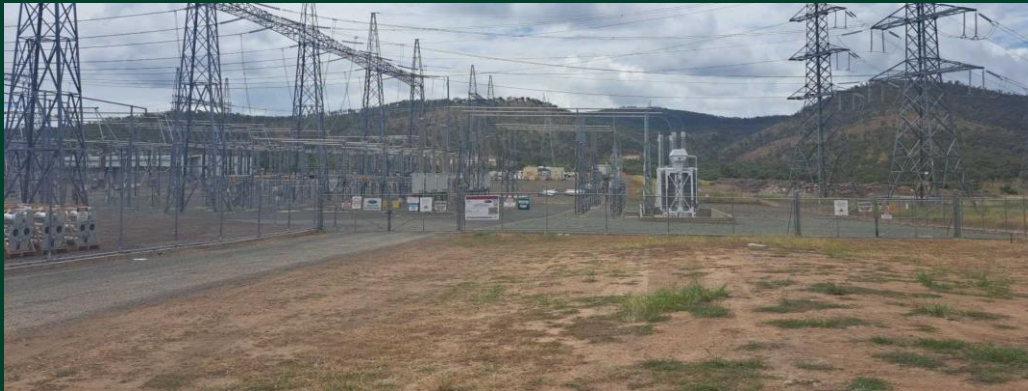
Powerlink Substation – 08/03/2023 Internal Use
